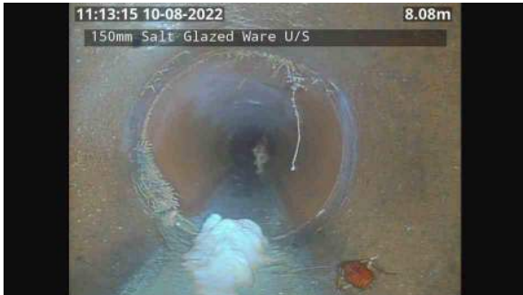
LS163731_d0ede370-bea8-4cd3-9b08-c4b84951a1a0_20220809_111356_762.jpg, 00:16:35, 8.08 Multiple/complex wall crack, at joint, width: 2mm from 12 o'clock to 12 o'clock
