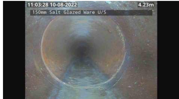
LS163731_d6ff81f3-369f-4d07-92b9-8a8a29aaa666_20220809_110410_133.jpg, 00:08:18, 4.42 Multiple/complex wall crack, at joint, width: 2mm from 12 o'clock to 12 o'clock
