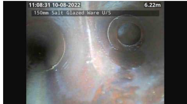
LS163731_83d94429-23f5-42aa-b19c-17e06b1a1b28_20220809_110932_065.jpg, 00:13:18, 6.22 Junction open, good workmanship, height: 100mm at 3 o'clock
