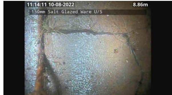
LS163731_49a33510-9e99-411f-b144-f42570773bad_20220809_111513_323.jpg, 00:17:54, 8.86 Multiple/complex wall crack, at joint, width: 2mm from 12 o'clock to 12 o'clock
