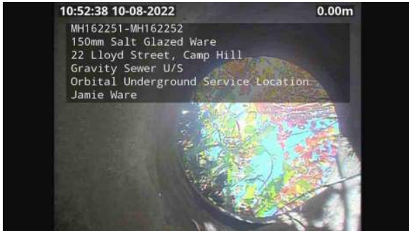
LS163731_2f00863f-889c-4e45-8962-94408b10f2db_20220809_105319_801.jpg, 00:00:00, 0.00 Start node, maintenance hole, Nodename:, MH162251
