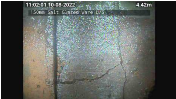
LS163731_4899ed5a-411c-4a0a-9496-ef50f0c96574_20220809_110301_328.jpg, 00:08:18, 4.42 Multiple/complex wall crack, at joint, width: 2mm from 12 o'clock to 12 o'clock
