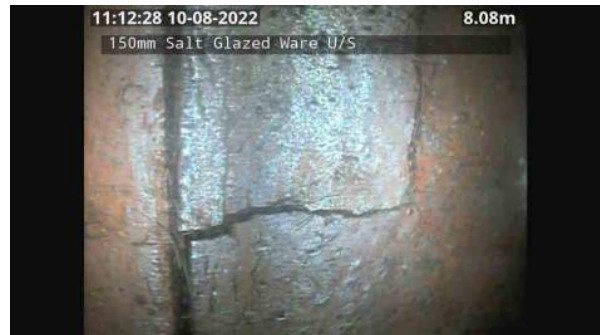
LS163731_cb244404-ceb0-4cba-91de-627f381839de_20220809_111331_281.jpg, 00:16:35, 8.08 Multiple/complex wall crack, at joint, width: 2mm from 12 o'clock to 12 o'clock
