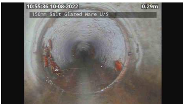
LS163731_ab50eb80-27a0-4926-8f2f-b0f3958cb291_20220809_105617_788.jpg, 00:02:11, 0.29 Multiple/complex wall crack, at joint, width: 2mm from 12 o'clock to 12 o'clock
