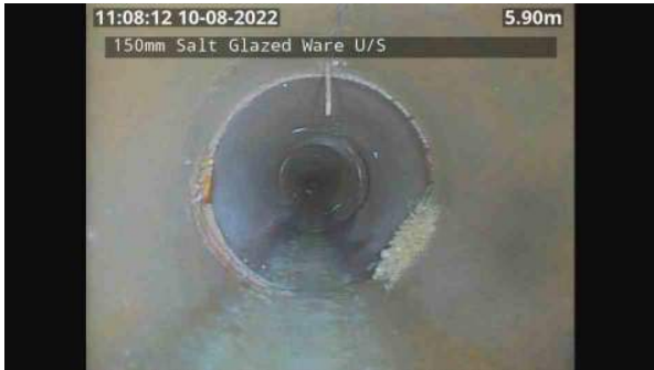
LS163731_33b182b9-f80b-4f3e-a7dc-07076401cc72_20220809_110854_610.jpg, 00:12:31, 5.90 Multiple/complex wall crack, at joint, width: 3mm from 12 o'clock to 12 o'clock
