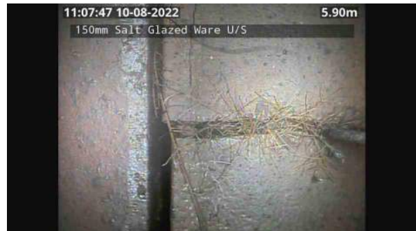
LS163731_de50a039-b529-4bd8-950f-8886be089dc2_20220809_110829_076.jpg, 00:12:31, 5.90 Multiple/complex wall crack, at joint, width: 3mm from 12 o'clock to 12 o'clock
