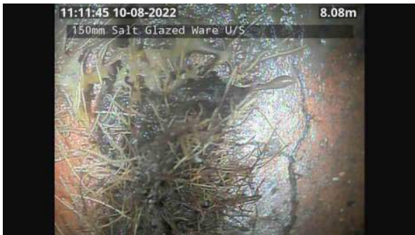
LS163731_3d29be1c-a4cb-4ba1-a4ee-8e62a1ced634_20220809_111243_413.jpg, 00:16:11, 8.08 Roots, at joint at 7 o'clock
