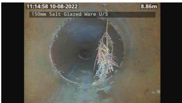
LS163731_21168ccc-f882-41c8-9dfa-e703e0e8c54c_20220809_111603_193.jpg, 00:18:19, 8.86 Roots, at joint from 9 o'clock to 4 o'clock
