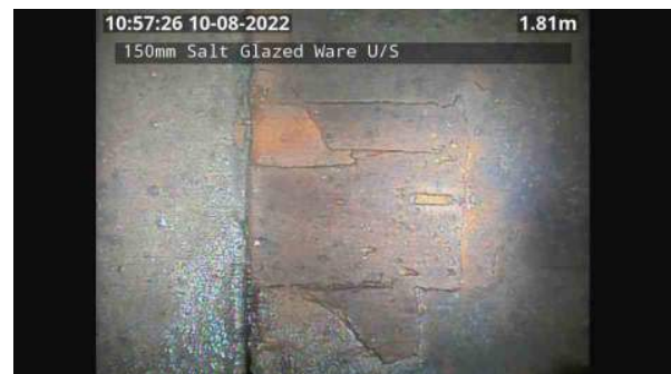
LS163731_bb5b977e-913a-4611-ab69-9c9242840279_20220809_105844_999.jpg, 00:04:22, 1.81 Multiple/complex wall crack, at joint, width: 1mm from 4 o'clock to 5 o'clock
