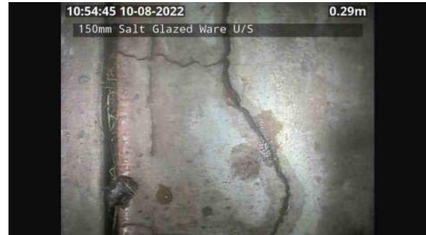
LS163731_fddb97a0-3fc1-423e-b3a3-909baecc66eb_20220809_105554_951.jpg, 00:02:11, 0.29 Multiple/complex wall crack, at joint, width: 2mm from 12 o'clock to 12 o'clock
