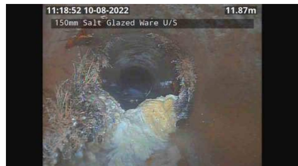
LS163731_fd38a73e-26f2-4cd0-b5c9-9c1e3bfb4db0_20220809_112002_539.jpg, 00:21:47, 11.87 Roots, 4) 20 - 40% of circumference, at joint from 12 o'clock to 12 o'clock
