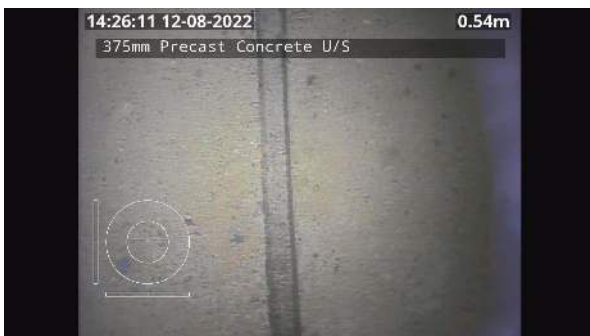
2_ccad764b-72a3-4b07-8223-4d4b797a7550_20220811_142712_039.jpg, 00:01:58, 0.54 Displaced joint, longitudinal displacement, longitudinal displacement: 10-20mm at 12 o'clock
