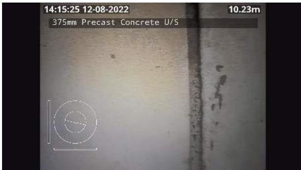
1_1f983942-07af-46bb-bb51-4a4a8a776d95_20220811_141627_952.jpg, 00:09:06, 10.23 Displaced joint, longitudinal displacement, longitudinal displacement: 10-20mm at 12 o'clock
