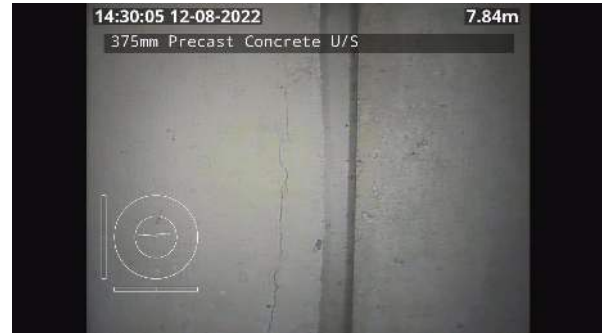
2_86d8aeb3-9bf2-4faa-9b34-8e133b939c95_20220811_143110_651.jpg, 00:05:01, 7.84 Circumferential wall crack, at joint, width: 1mm from 11 o'clock to 1 o'clock
