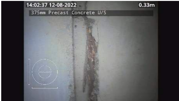
1_6b540bfc-e687-4be2-911c-c8dc1e484ca1_20220811_140459_056.jpg, 00:02:05, 0.33 Steel reinforcement is visible and projecting into the conduit, at joint from 9 o'clock to 5 o'clock
