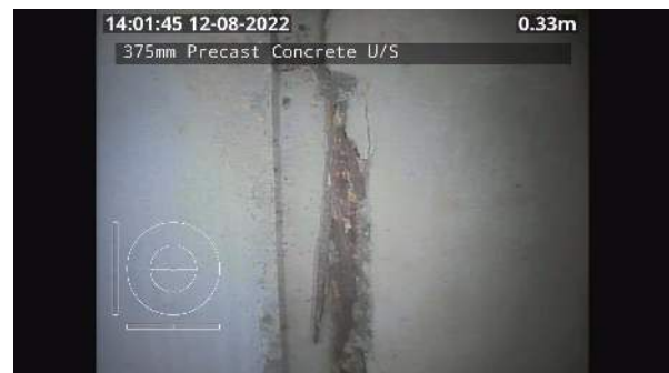
1_640bf76d-9fac-40bf-b8b1-c9247a7c5d5e_20220811_140313_540.jpg, 00:02:02, 0.33 Displaced joint, longitudinal displacement, longitudinal displacement: >30mm at 12 o'clock
