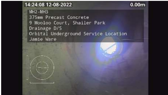
2_a1ccb371-f6f2-41b6-9916-f0905a8550a7_20220811_142450_746.jpg, 00:00:00, 0.00 Start node, maintenance hole, Nodename:, MH2
