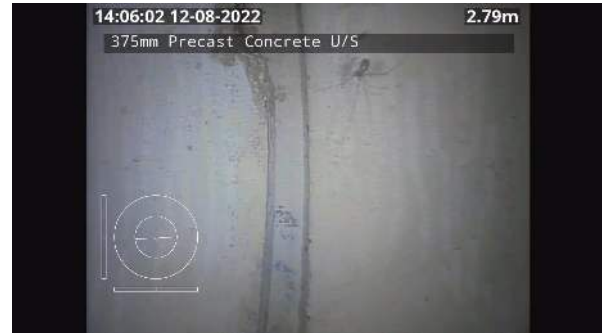
1_609d39c6-3de4-4952-b427-81ec529ef3f0_20220811_140725_863.jpg, 00:03:48, 2.79 Displaced joint, longitudinal displacement, longitudinal displacement: >30mm at 12 o'clock
