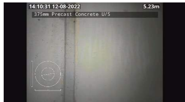
1_e141f3d4-8ddd-4fb3-a2ac-7b4198ba411e_20220811_141132_172.jpg, 00:06:00, 5.23 Displaced joint, longitudinal displacement, longitudinal displacement: 21-30mm at 12 o'clock
