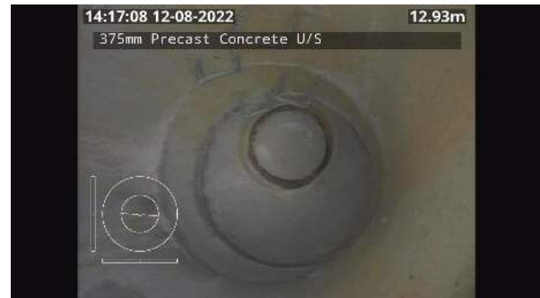
1_1d845ed1-0190-4290-b800-888ec4aacf67_20220811_141751_201.jpg, 00:10:10, 12.93 Finish node, maintenance hole, Nodename:, MH1
