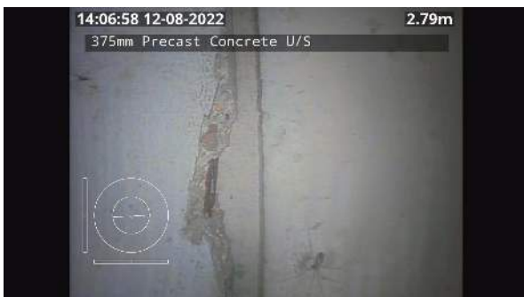
1_7b1e371c-4a57-4159-8b7e-25aba316bc81_20220811_140911_870.jpg, 00:04:01, 2.79 Breaking, some pieces are missing, at joint, length of break: 100mm at 2 o'clock / Broken spigot
