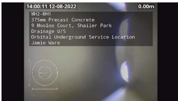
1_bc7360f2-6c4f-4518-b05d-6f5037d6a297_20220811_140054_291.jpg, 00:00:24, 0.00 Circumferential wall crack, width: 2mm from 12 o'clock to 12 o'clock
