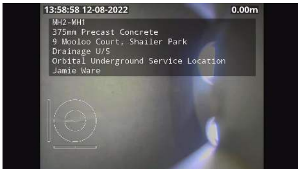
1_b851db90-8355-4dd8-869b-627495cf1608_20220811_135941_021.jpg, 00:00:00, 0.00 Start node, maintenance hole, Nodename:, MH2
