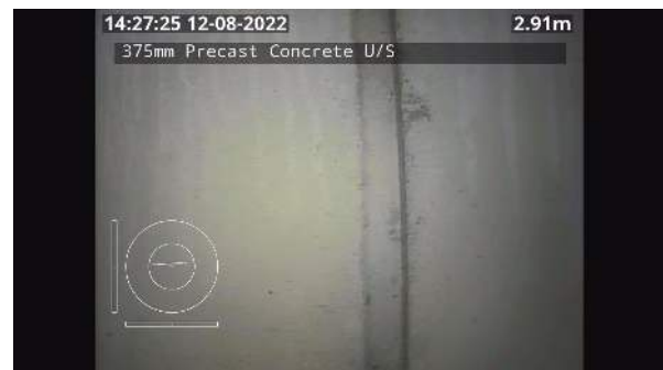
2_a5729d3b-4510-4955-8516-465be0dd0164_20220811_142822_015.jpg, 00:02:52, 2.91 Displaced joint, longitudinal displacement, longitudinal displacement: 10-20mm at 12 o'clock
