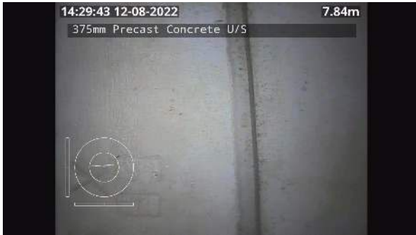
2_84634ada-02b3-4ee7-84fd-36fca8b637e2_20220811_143040_353.jpg, 00:04:55, 7.84 Displaced joint, longitudinal displacement, longitudinal displacement: 10-20mm at 12 o'clock
