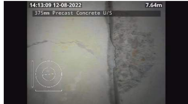
1_7cc0c38b-218b-4f9a-900d-23252f57c2ed_20220811_141420_824.jpg, 00:07:52, 7.64 Longitudinal surface crack, at joint, width: 1mm at 9 o'clock
