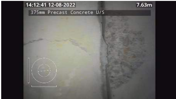
1_1a7c3295-c7ce-4524-89e3-7b3c108df658_20220811_141346_311.jpg, 00:07:49, 7.49 Breaking, some pieces are missing, at joint, length of break: 100mm at 9 o'clock
