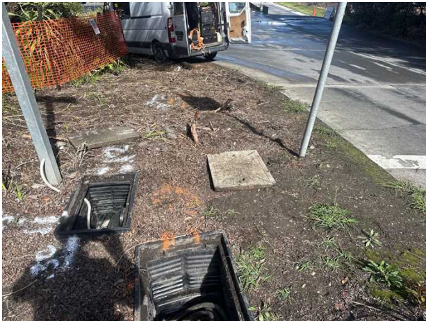
Electrical asset. Four conduits running down the hill, stacked two on two, at approximately 550mm (top conduits) and 750mm (bottom conduits). Classified as QL-B.
