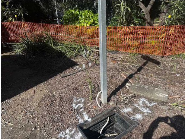
Communications asset. There are two conduits here that are 550-710mm deep, as marked. Located by electromagnetic field locator (EMF) techniques. Classified as QL-B.
