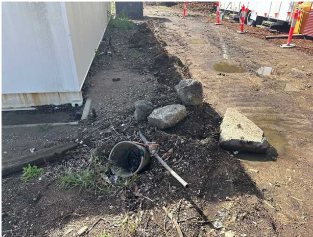
Water main/pipe. There is some irritation piping above ground here and it's in disrepair. Alignment established by site features. Classified as QL-D.
