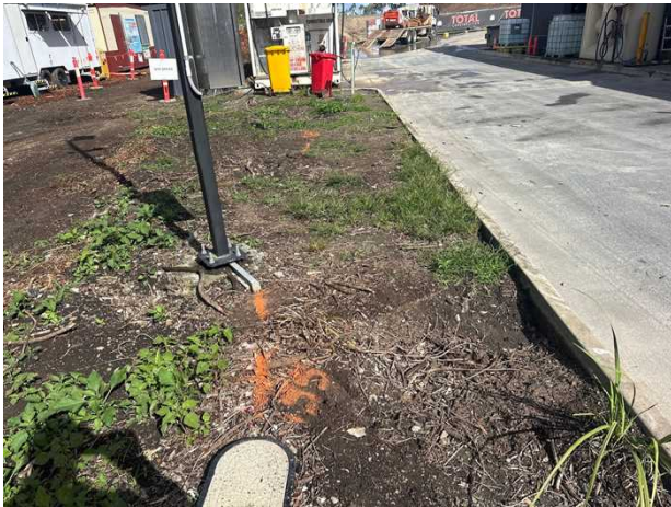
Electrical asset. One cable runs to this post after exiting the pit at 550mm deep and the other continues to the fuel storage at approximately 580-720mm deep. Located by electromagnetic field locator (EMF) techniques. Classified as QL-B.
