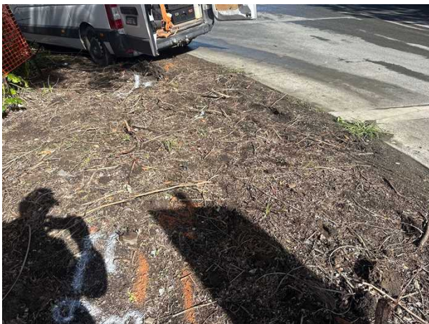
Electrical asset. This is the same conduits here at 940mm and then bear the roadway at approximately 610mm, where one set goes straight ahead and the other turns to the left under the roadway. Located by electromagnetic field locator (EMF) techniques. Classified as QL-B.
