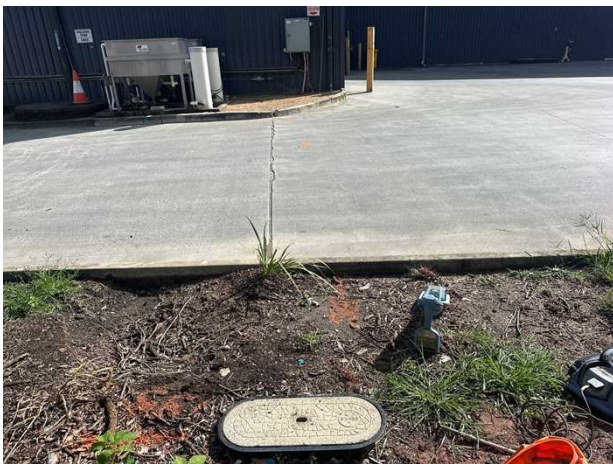
Electrical asset. The cable crosses into the pit at 550mm deep from the other side of the roadway, crossing at approximately 690mm deep. Located by electromagnetic field locator (EMF) techniques. Classified as QL-B.
