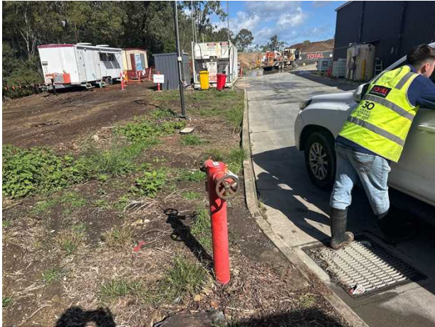
Fire Service. This stand pipe will link up with the stand pipe opposite the fuel storage. I can't trace this pipe without the fuel being moved. Alignment established by site features. Classified as QL-D.
