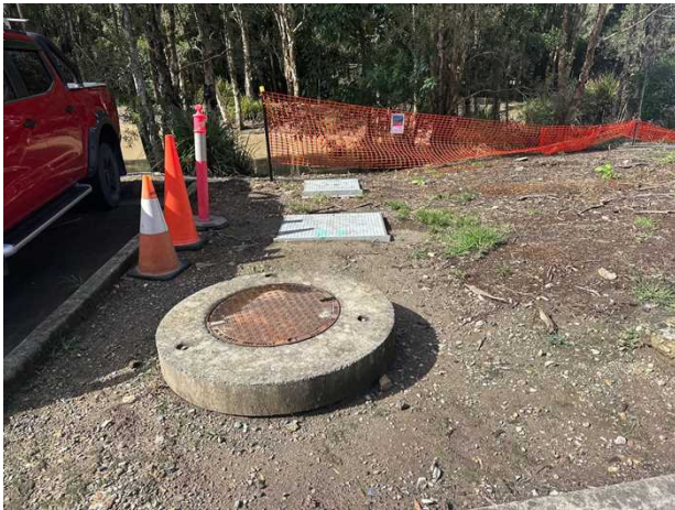
Drainage pipe. The drainage runs from the manhole, through silt catchers, to the dam. Alignment established by site features. Classified as QL-C.
